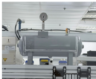
Gambar 4. Air Tank Booster
